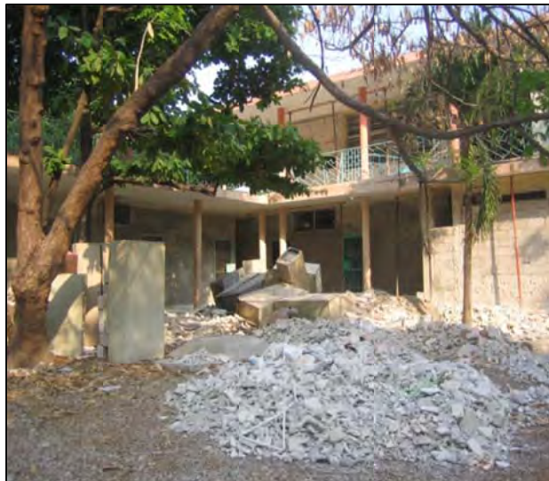
Earthquake damage to Ministry of Agriculture, Natural Resources, and Rural Development offices in Port-au-Prince.
